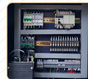
Electric control cabinet
